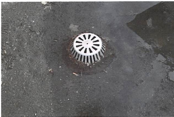
Debris in drain.
