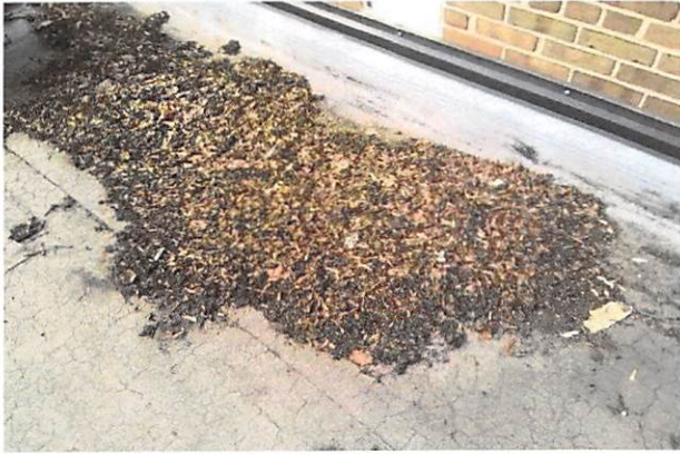
Debris on roof.
