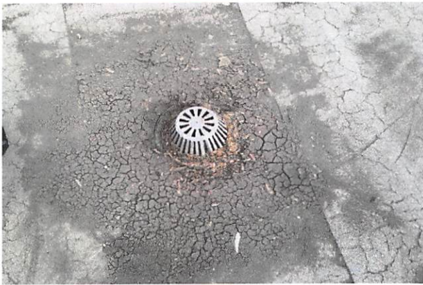
Debris in drain.
