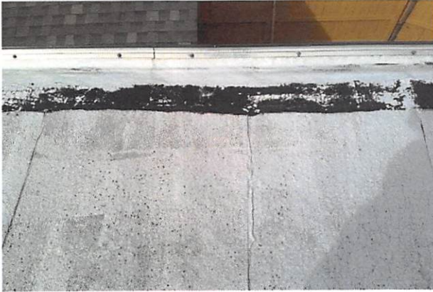
Weathered perimeter flashing.
