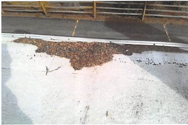
Debris on roof.
